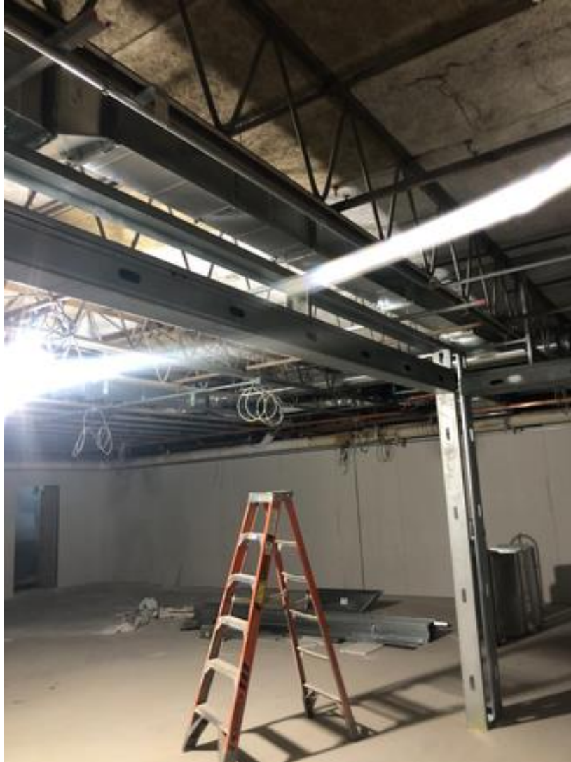
Sheetrock and framing ongoing in Media Center. This area will have the operable partition
