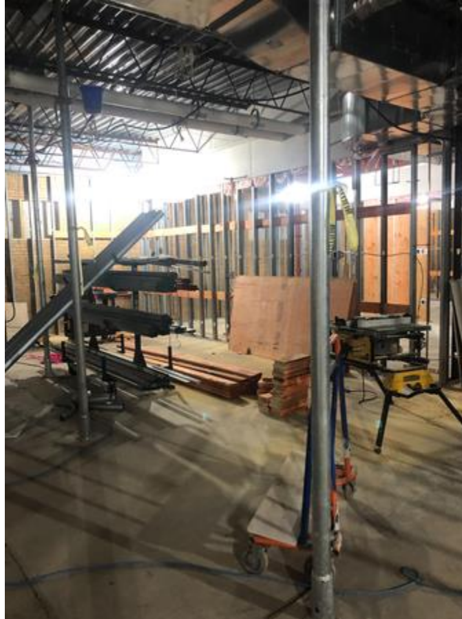
Steel stud framing and plywood backer ongoing. This area is the future “Flex Space”
