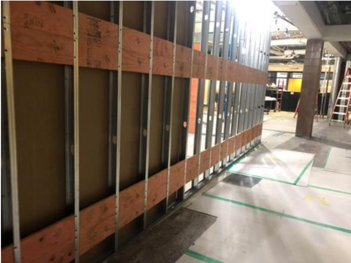
Steel stud framing finishing up. In-wall backing going in for lockers, digital displays, etc.
