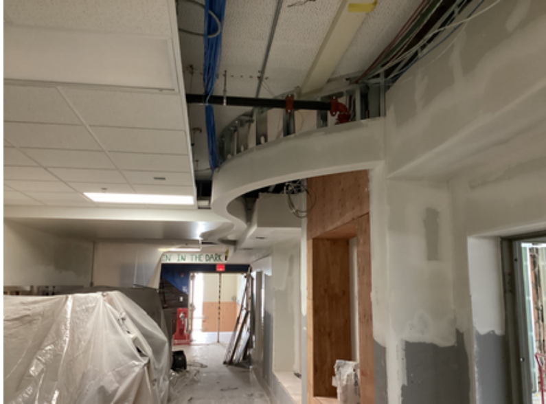
Soffits and wall framing for flex nooks and display case outside science classrooms.
