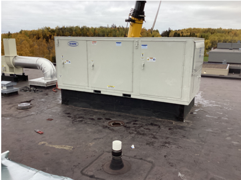
Roof top mechanical unit installed above science room
