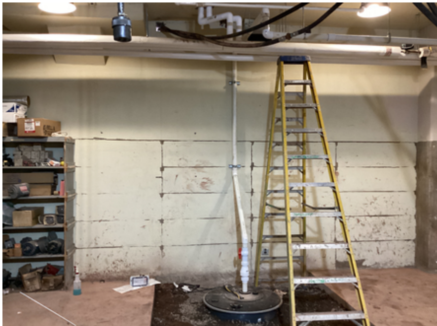
Sump pump installation
