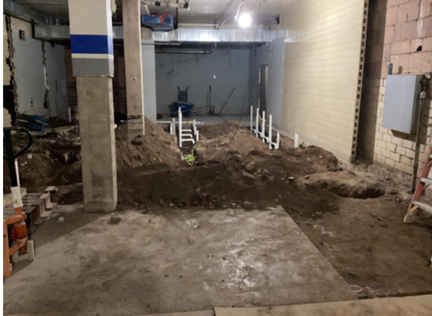
Underground plumbing in boys' locker room
