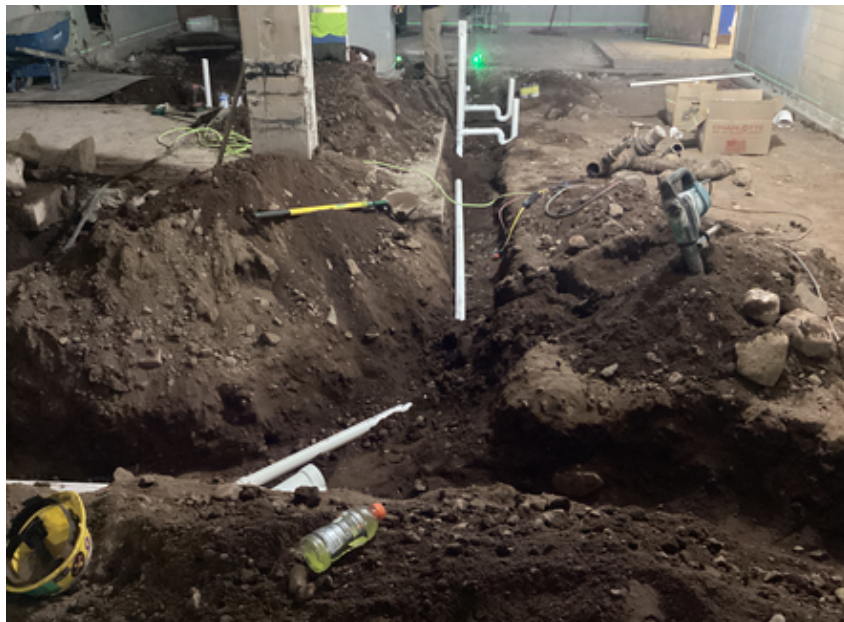
Underground plumbing in boys' locker room
