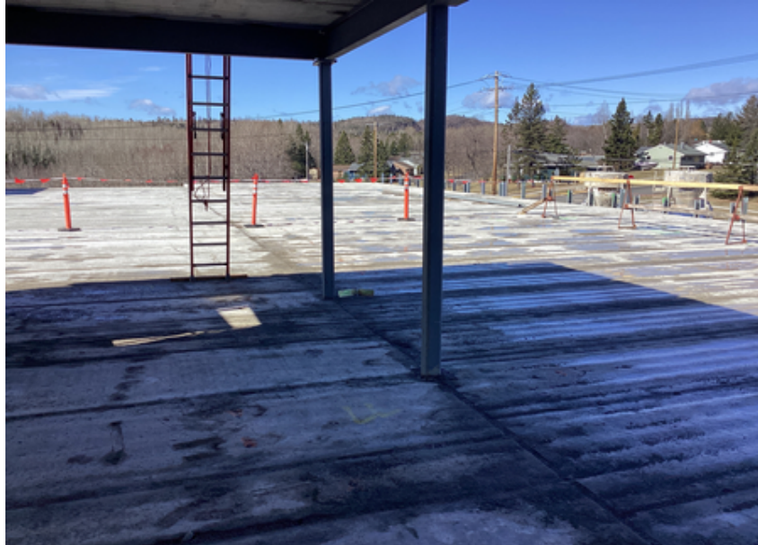
Precast plank grouting and additional steel framing at Area B Music Suite
